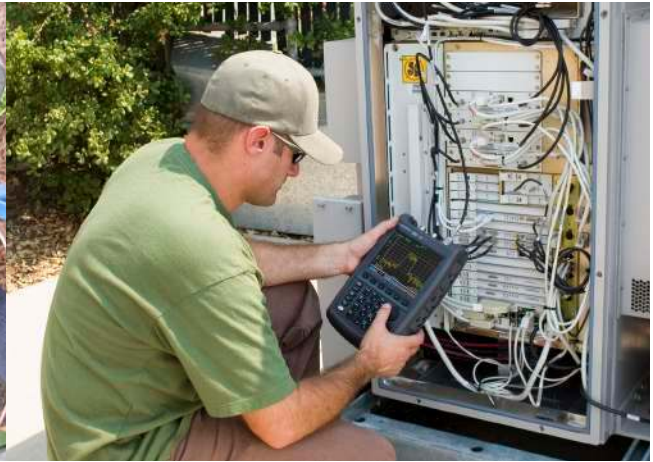
Figure 1b. FieldFox directly connected to a feeder line on a wireless communication system
