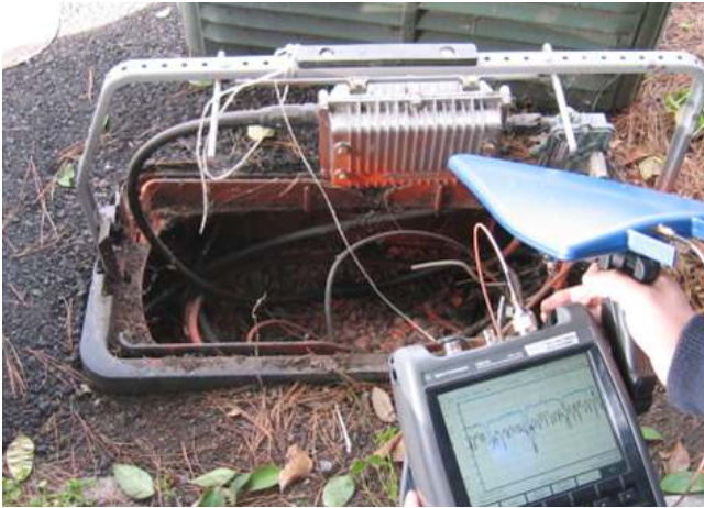
Figure 1a. FieldFox connected to a directional antenna for locating a source of radio interference
